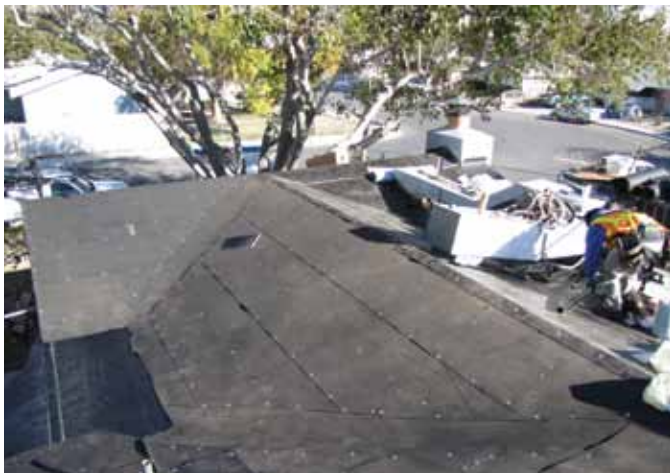
Commercial Roofers reroofs the home of Jack Brown, a disabled veteran, in Las Vegas.
